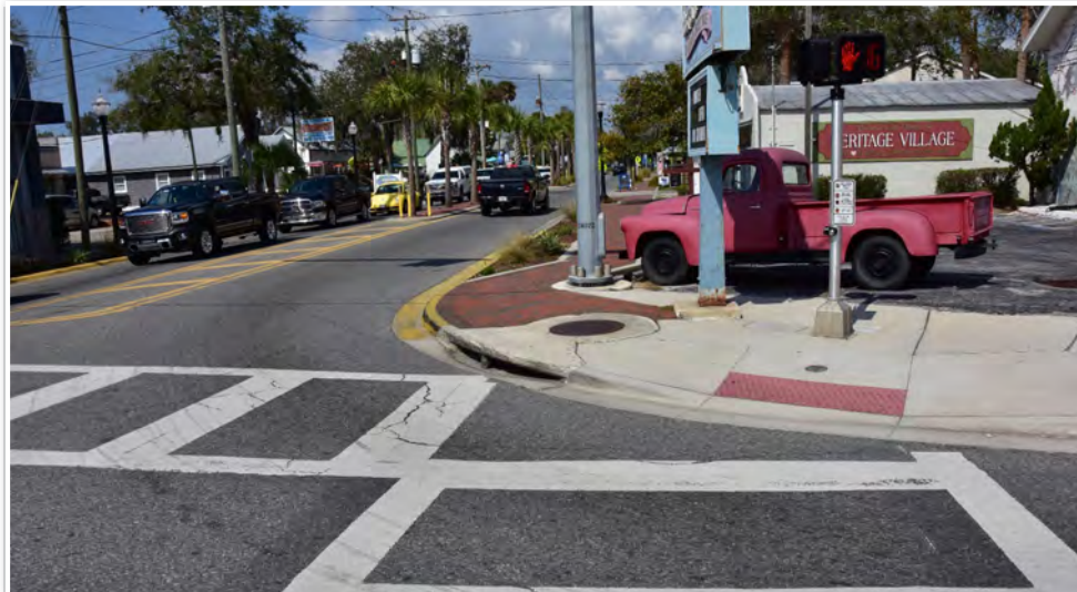
Northeast corner of US 19 at Citrus Avenue looking north showing tire scuff marks on the curblines and drainage inlet.
